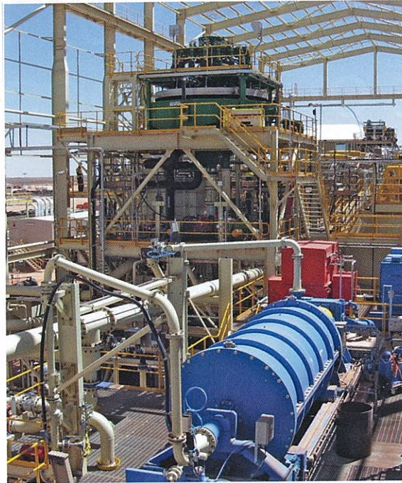
At Prominent Hill, a rougher concentrate is reduced from over 100µm to 24µm by a M10,000 IsaMill, and is then treated by a Jameson Cell
